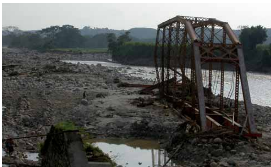
Environmentally-driven threat: tropical storm Stan damage in Guatemala
